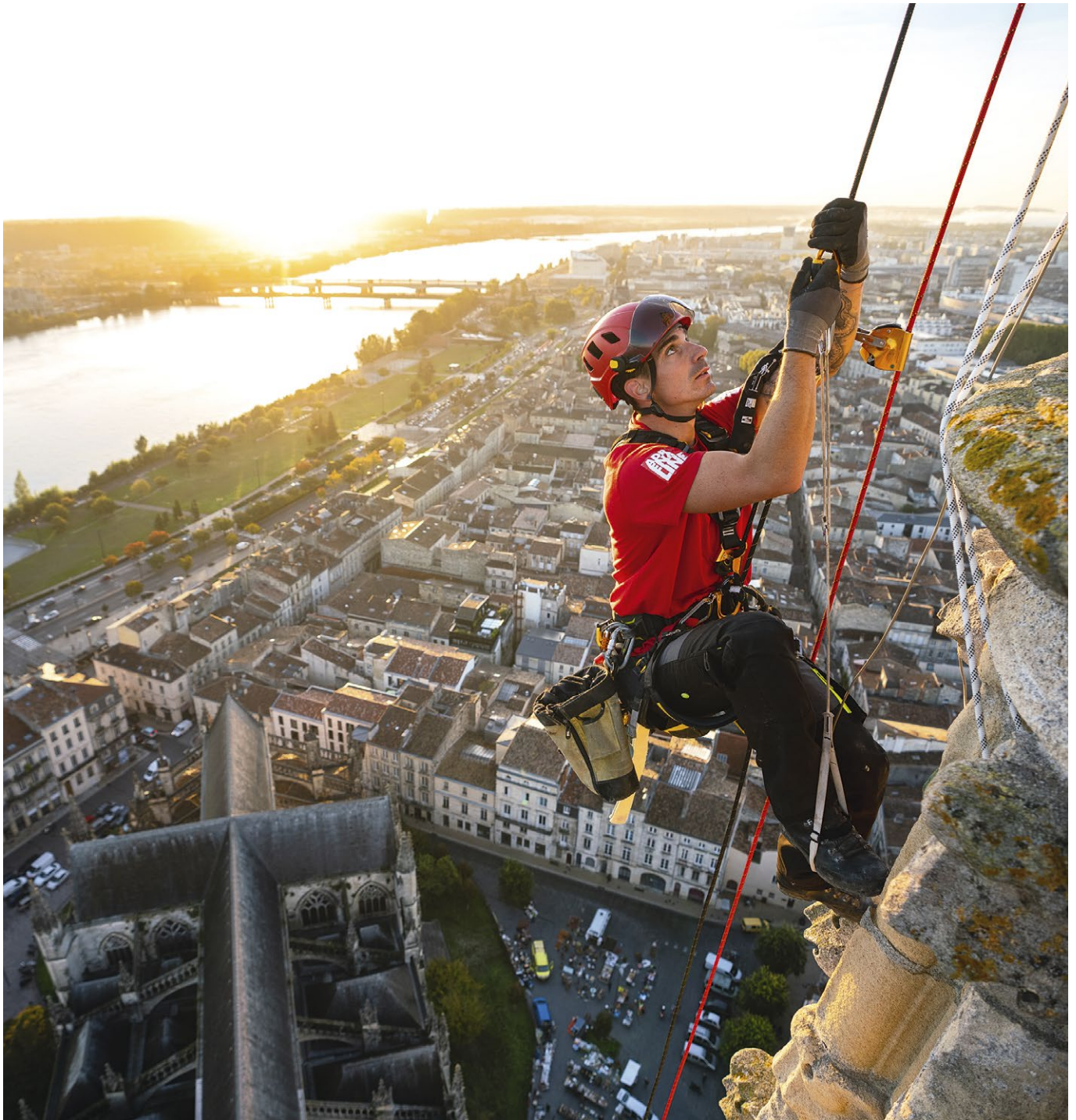
Installing monitors on the spire of the St Michel Church, Bordeaux, France © 2021 Petzl Distribution - Vuedici.org - Adréaline - Bordeaux City Hall
